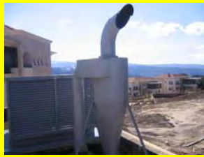
Hot air & exhaust outlets
